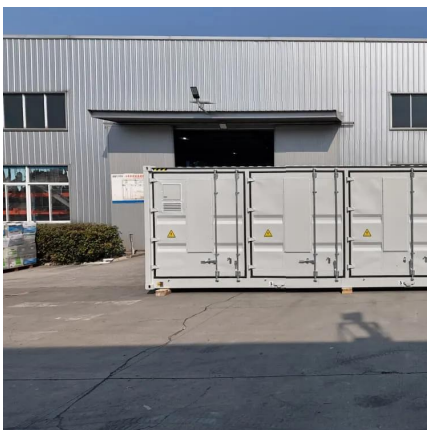
GSL 5MWh Battery Energy Storage System
