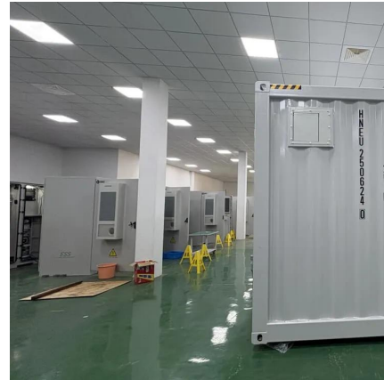
Solarcontainer: The mobile solar system
