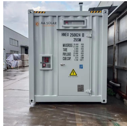
Solar Battery Container
