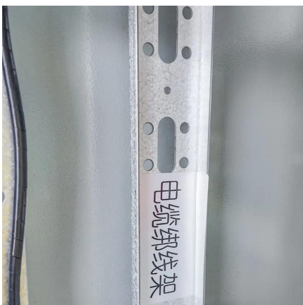
Battery Energy Storage Containers: Mobile Solar Power ...
