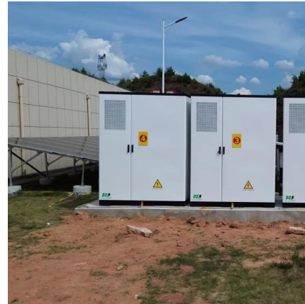
Energy storage container , SCU , energy ...
