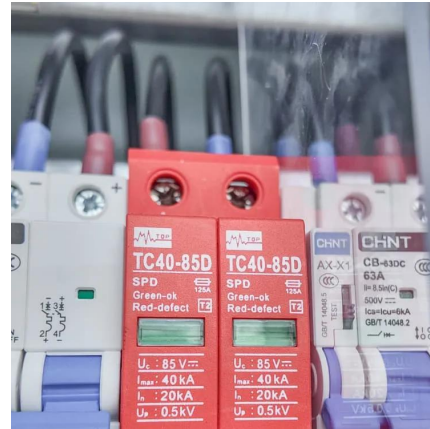
Battery storage power station - a ...
