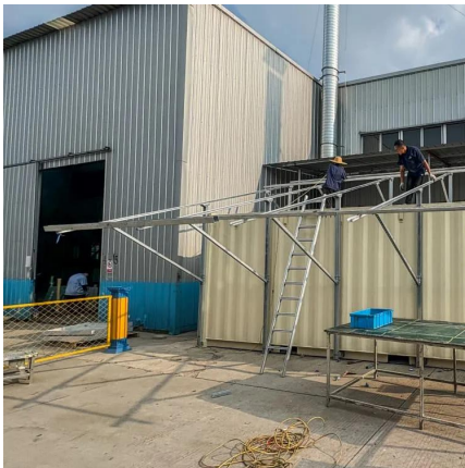
Solarcontainer: The mobile solar system
