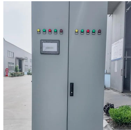
30KW 50KWH battery sytem container
